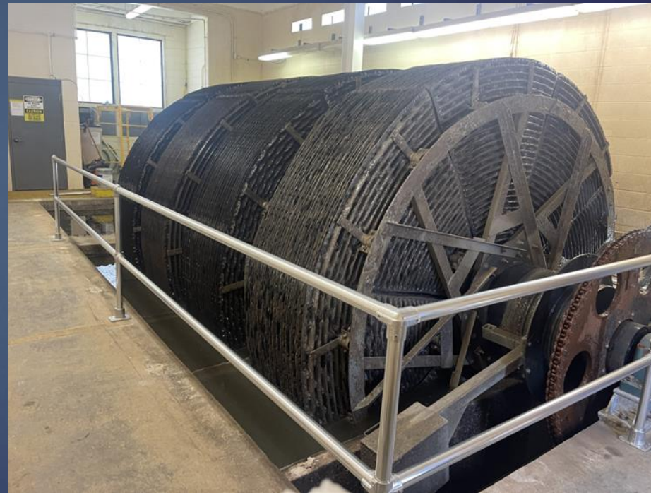
Rotating Biological Contactor (RBC) in Bridgewater, Vermont, Design Capacity of 35,000 gpd
